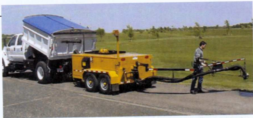
Spray injection units allow a contractor to repair a pothole without the labor of shoveling mix.
