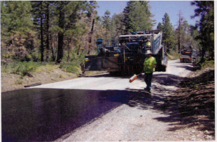
Narrow roads had to be closed and the chip sealing application modified in order to cover the full width of the road in one pass.
